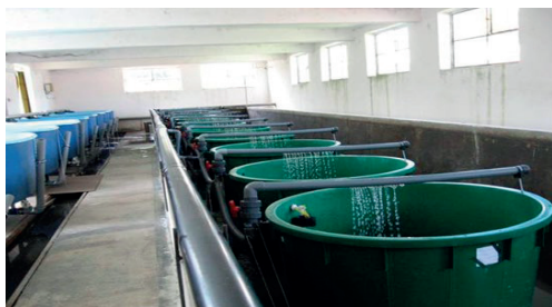
Figure 1. Pilot installation ("Evos" type basin) for raising and the development of pikeperch larvae in the post-embryonic period
