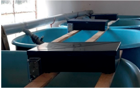
Figure 3. Automatic belt feeders (original photo)
